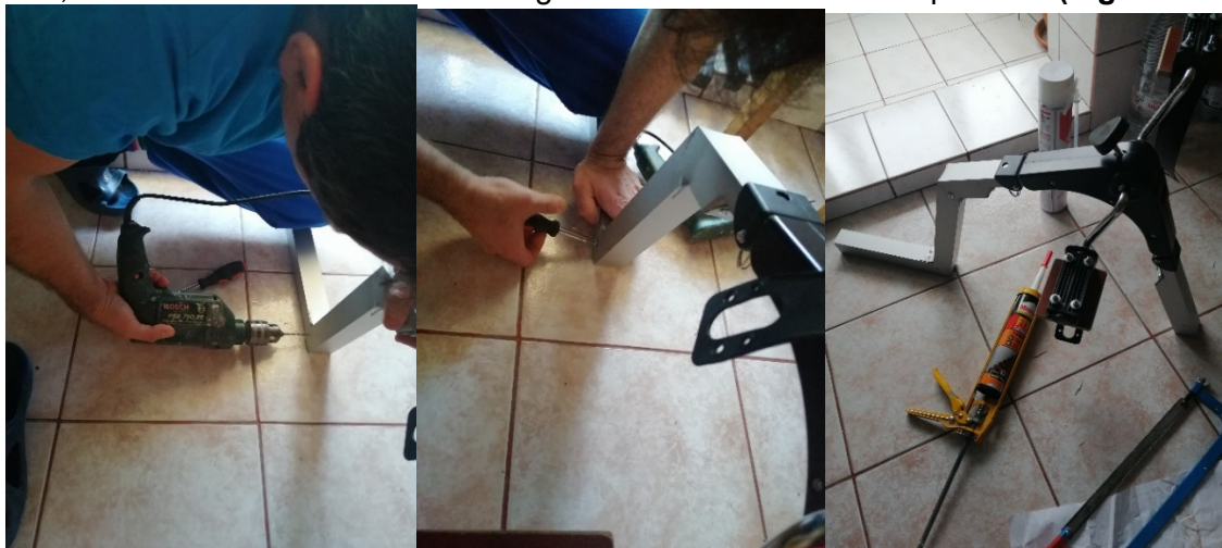
Figure 7.18 Fixing the angles of the aluminum profile with self-tapping screws for sheet metal [own contribution]
